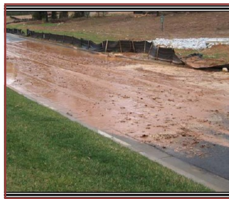
Example of Poor Erosion Control
