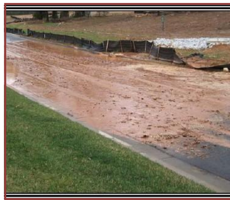
Example of Poor Erosion Control
