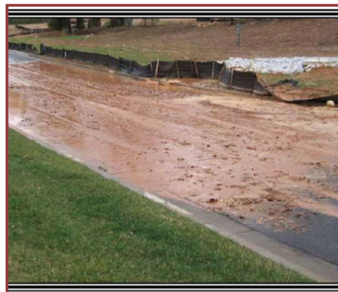
Example of Poor Erosion Control
